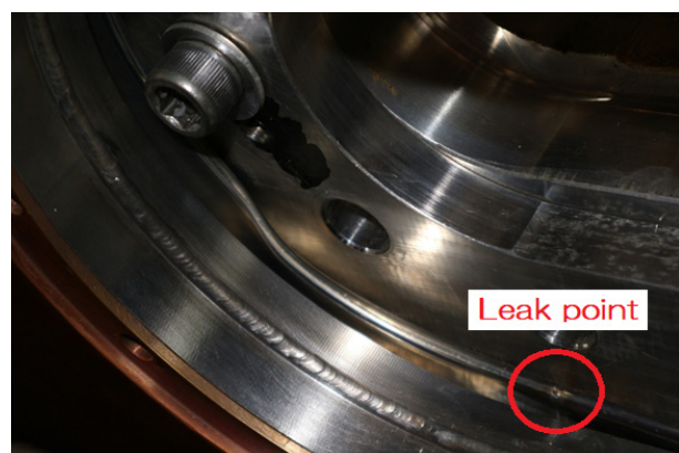
Figure 1: A leak point of the bellows for RRC #2.
