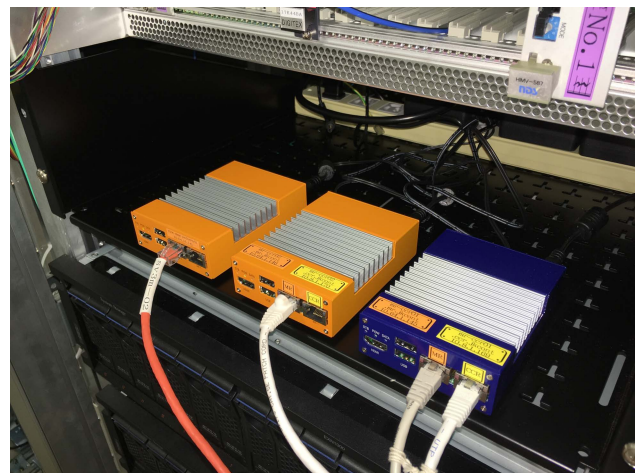
Figure 2: Three sabataros placed on a 19 inch rack shelf.
