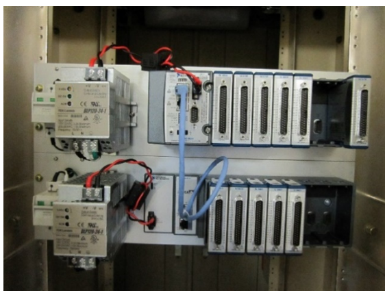
Figure 5: CompactRIO under installation. The light blue cable is used in order to interconnect the EtherCAT slave chassis (down) to the EtherCAT master controller (up).
