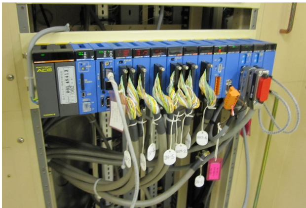
Figure 4: Consolidation of front-end computers. Left most is a power supply module (double width). Next to its right is an ordinary CPU module which runs ladder programs. Next to its right is the F3RP61 CPU module which functions as an IOC.
