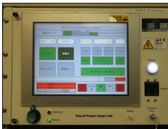
Figure 3: Automatic startup by the control system.
