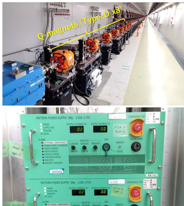
Figure 6: Photographs of the installed Q Type-D magnets in the matching section (Upper), and the pattern PSs (Lower).
