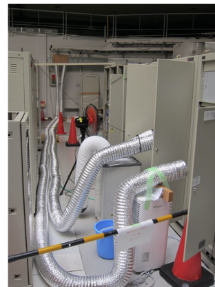
Figure 5: Cooling the bending magnet power supply with spot coolers.
