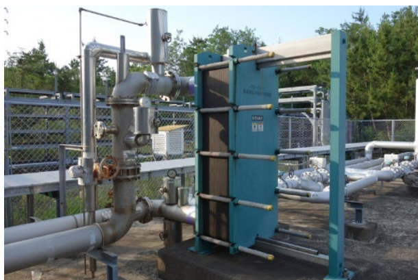
Figure 5: Heat exchanger HE-D1-1.
