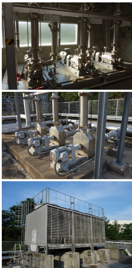
Figure 2: Pure water pumps PPW-D1-1-1~3 (upper), equipment cooling water pumps PCD-D1-1-1~3 (middle), and cooling towers CT-D1-1-1~3 (lower).
