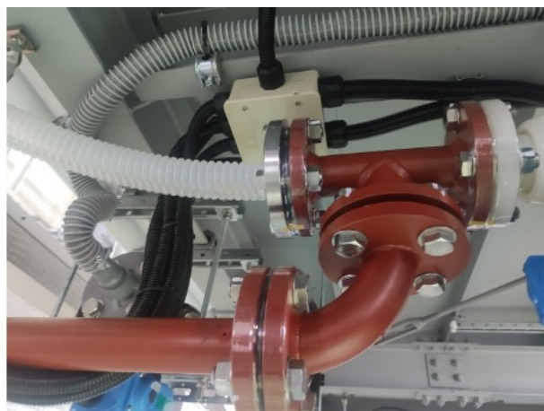
Figure 3: PVC film cover installed on the electrolyte piping flange connection.
