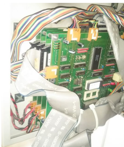
Figure 5: Photograph of personnel key system control board.
