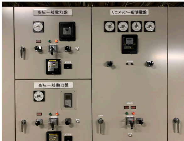
Figure 7: Photo of the high voltage switchgear where the analog indicating meters will be replaced. Replace one of the multiple analog indicating meters installed in the high voltage switchgear with a digital multimeter. By replacing one analog indicating meter with the digital multimeter, multiple values, such as power, power factor, etc., can be monitored simultaneously.
