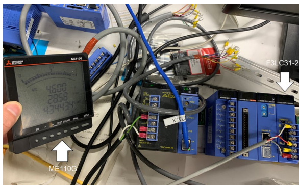
Figure 6: The situation in which F3LC31-2F is connected to ME110G and Modbus RTU communication is being tested.
