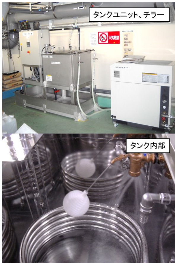
Figure 2: Upper: the tank unit and the chiller. Lower: Inside the tank.
