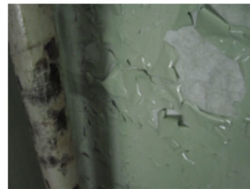
Figure 2: Peeled epoxy coating at \mu -monitor.
