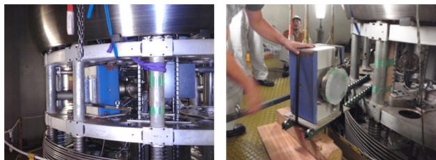
Figure 11: Removal of ion pump from dead section.
