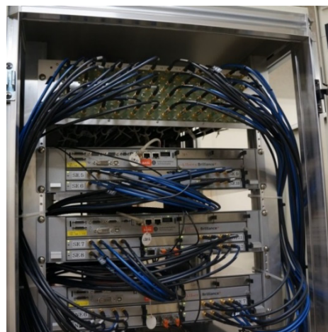
Figure 4: A part of the new beam position circuits installed into the standard 19 inch rack. Low loss 8D-size cable connects between each electrode and the panel on the upper part of the rack. A 2U-height box contains four detection circuits.
